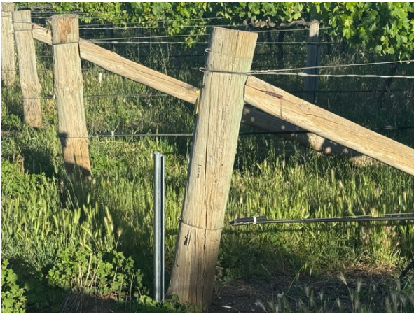
Place Ocloc SR behind the broken strainer ram into place with petrol rammer or sledge hammer.
