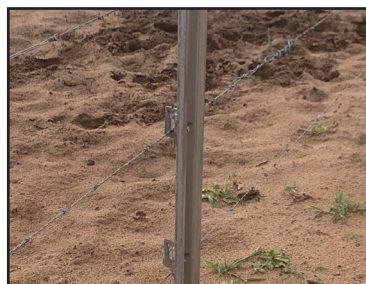
Rogue Buffalo Clip RBC after buffalo goes through the fence barb wire is easily reinstalled
